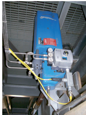
Metso B-series actuator at customer heater damper control
